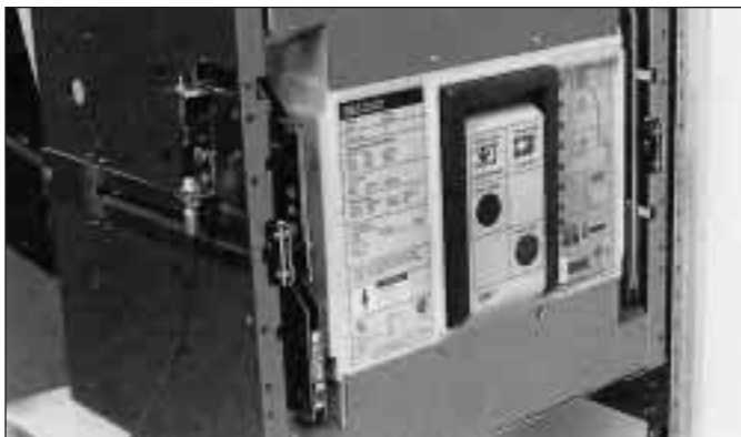
Dead Front Shields Installed
