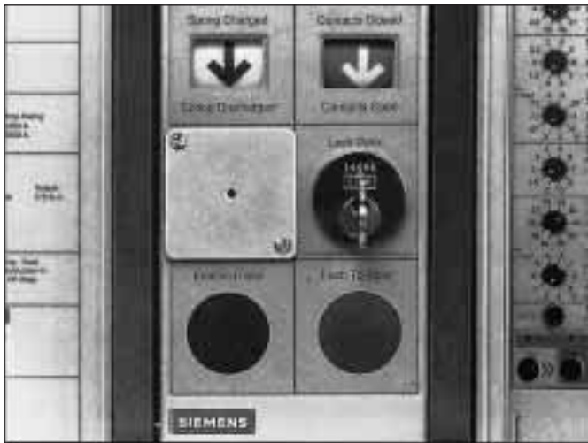
Closing Breaker Device is installed over the closed pushbutton switch.
